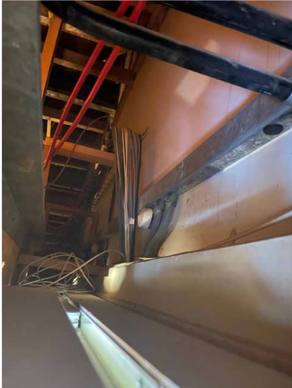
Figure 5.2 Photograph above the suspended ceiling in the Outer Hall, showing that the decorative ceiling does not survive.
